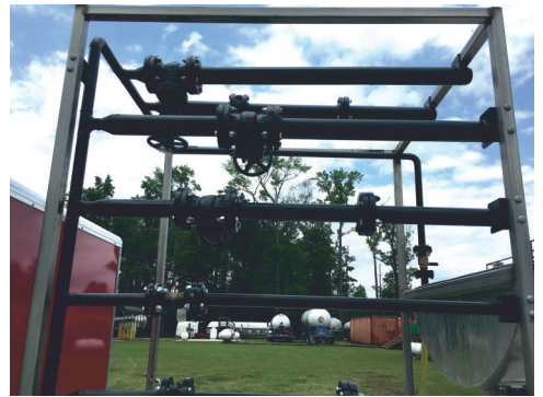
Sidewall Pipe Leaks
