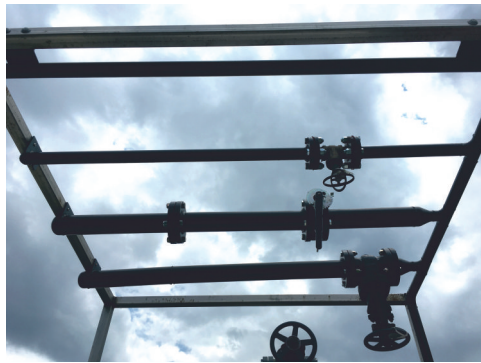
Overhead Pipe Leaks
